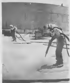
SHEETS ARE sandblasted prior to coating with Dometal to increase protection against corrosion.
